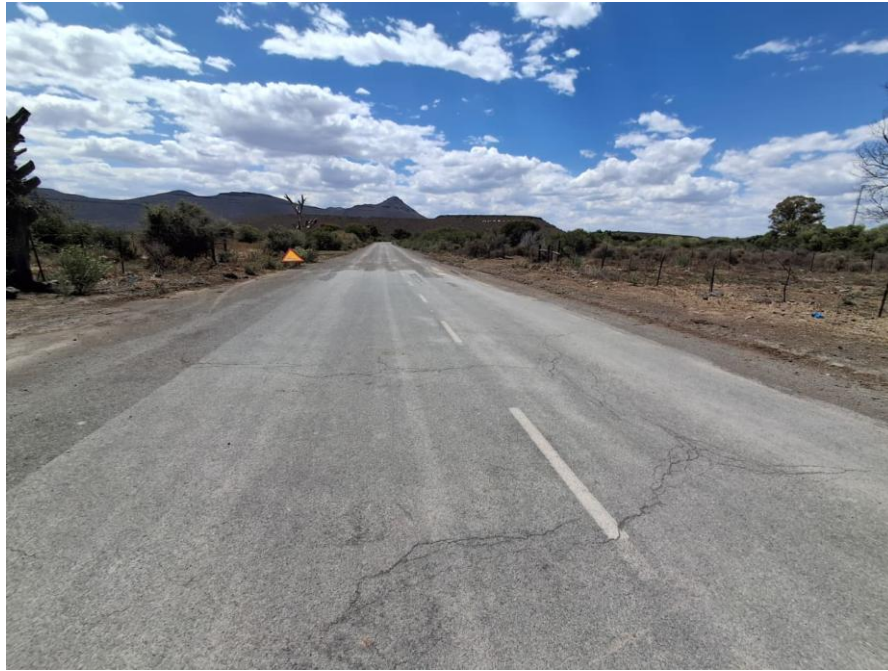
Figure B.6: Start of the MR00607 road in Murraysburg, showing the typical condition of the road (Source: CSIR, 2026)
